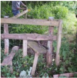
Old stile before replacement
